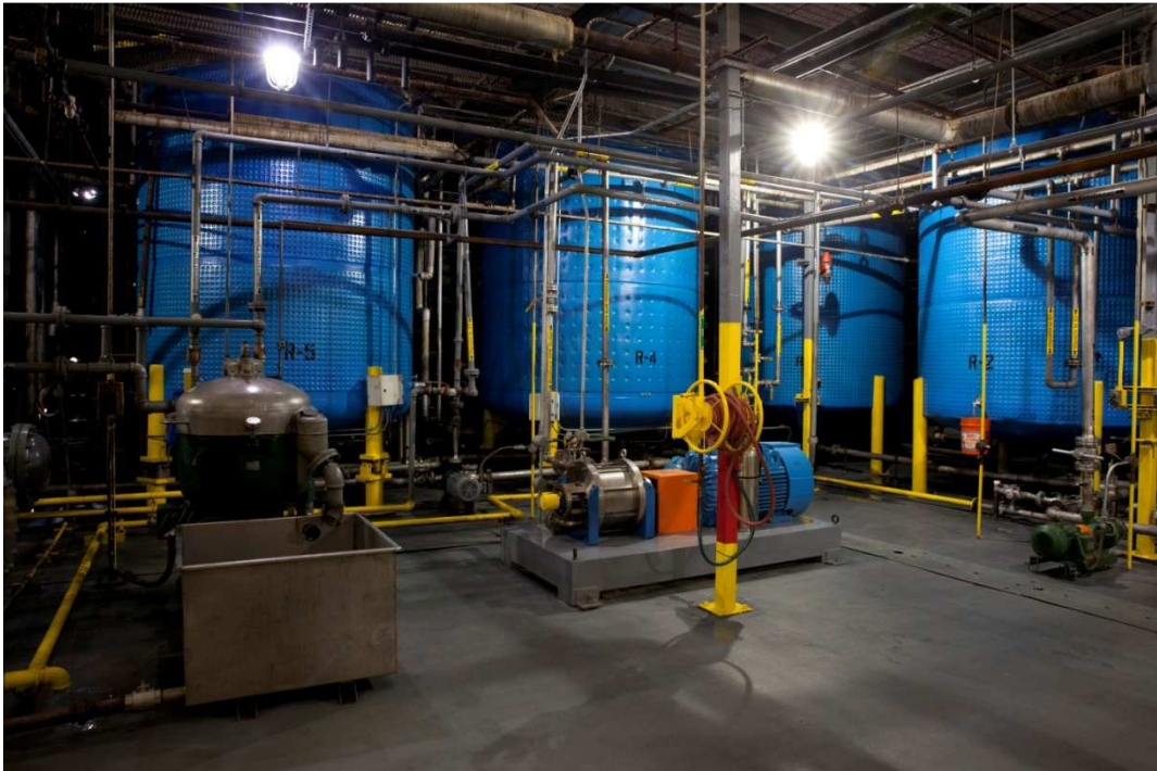
ShockWave Power Reactor installed in biodiesel plant.
