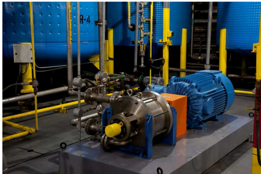
SPR Biodiesel Reactor
